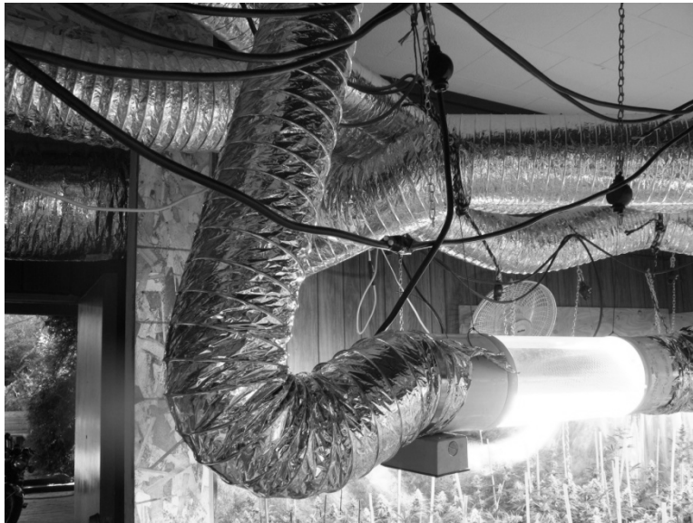
Figure 3: Photograph of ventilation tubing and electrical cords found in a residential IMC room
