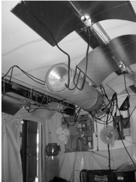
Figure 2: Photograph of overhead grow lights and electrical cords found in a residential IMC room
