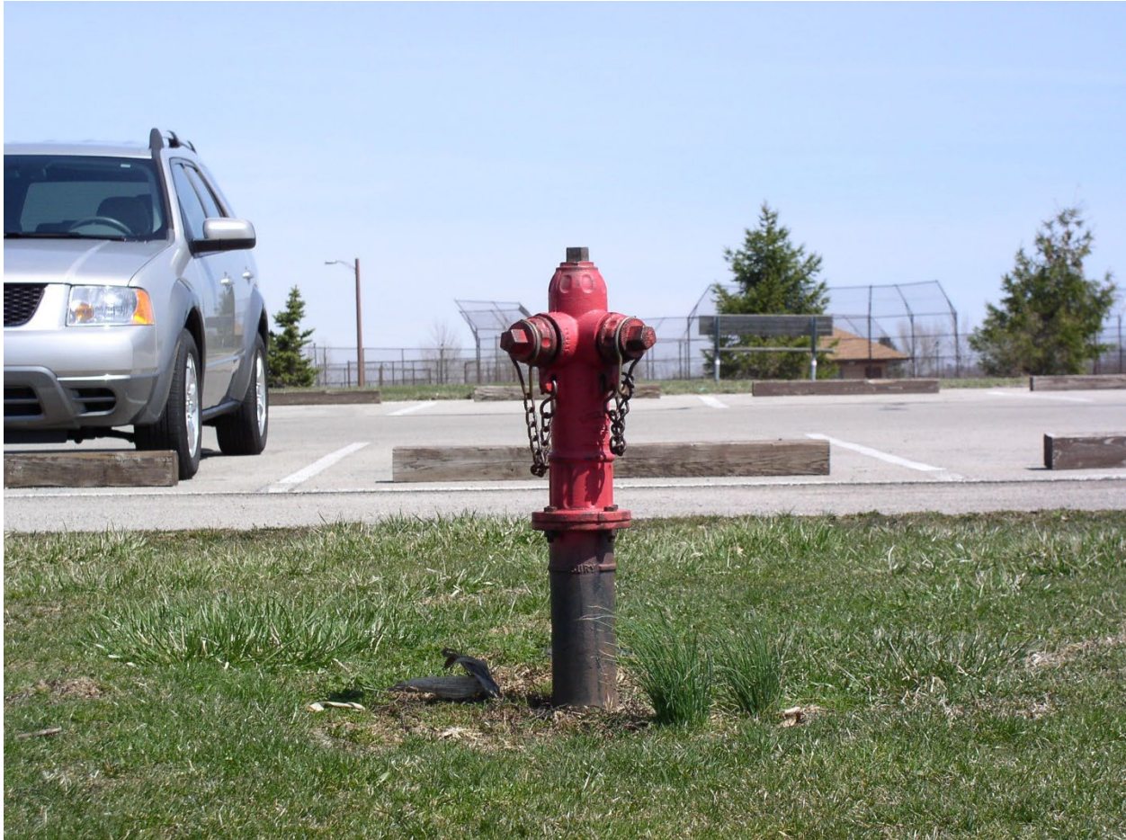
Figure 37. Municipal hydrant on edge of system.
