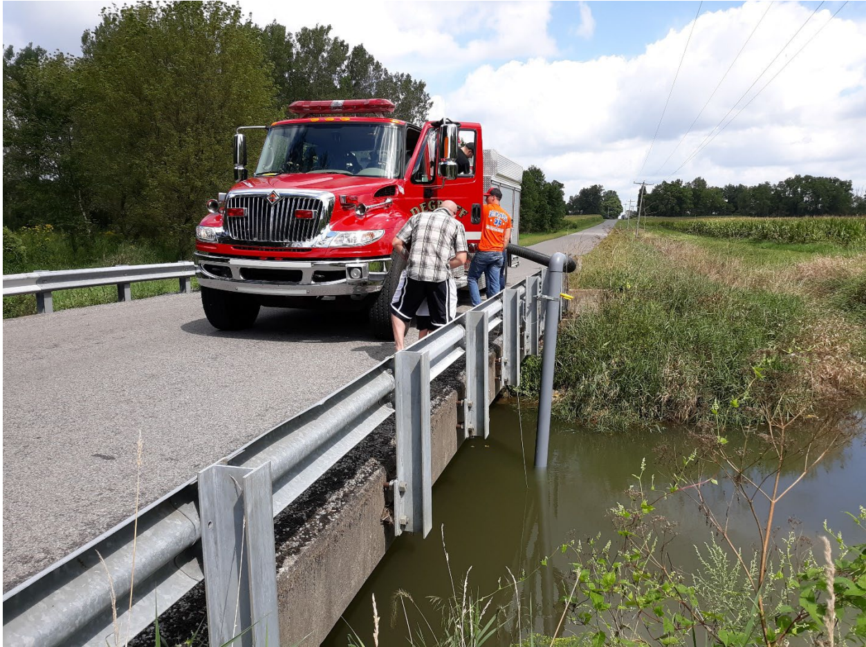
Figure 36. Bridge-mount dry hydrant in the study area.
