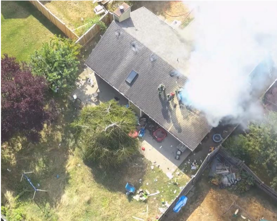
Figure 3: UAS View of Structure Fire, 8/20/2017, 9231 19 th Pl, SE, Lake Stevens, WA, (SCFD 22, 2017)
