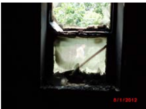
Broken window on south wall
