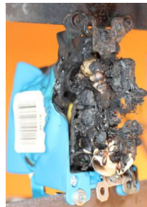
PVC receptacle – flaming faceplate melted and fell to floor.
