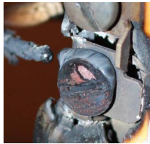
Severed conductor (welded with curved striations)
