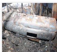
Lights destroyed approximate value $200
