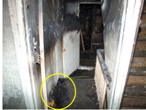
Multiple Fire Origins or Drop Down?
