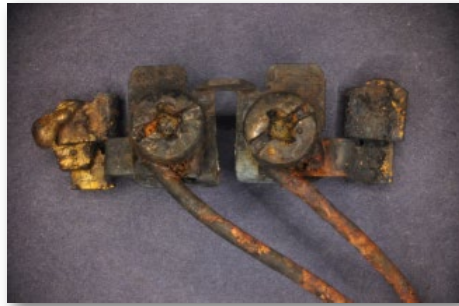
trolley power rail showing melted blade receptor and plug blade remnant.
