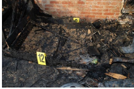
Love seat right by ventilation point
