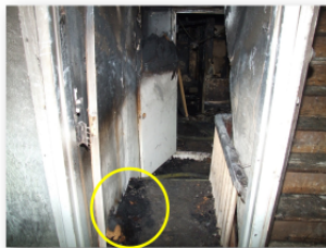
Multiple Fire Origins or Drop Down?
