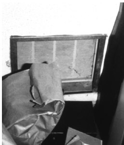
Return air vent
