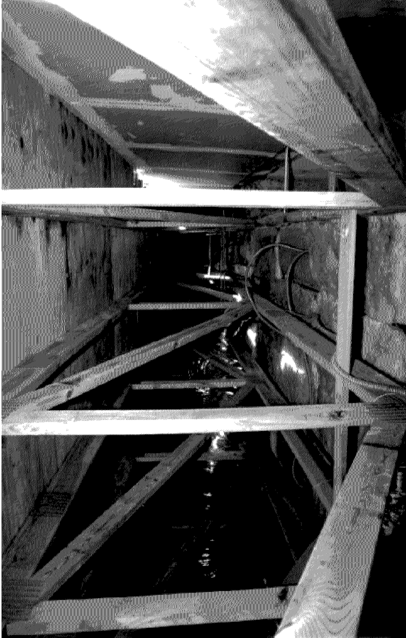
The truss loft area in another part of the Indian River Shopping Center. (Photo courtesy of the NFPA)
