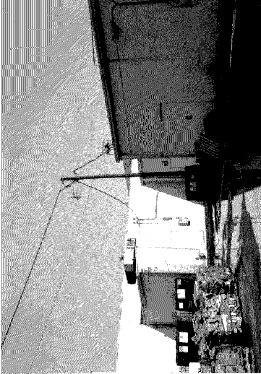
Utility pole connecting power to a meter at the rear of the Indian River Shopping Center. ( USFA file photo. )
